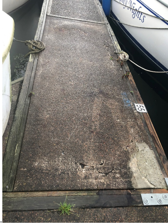
Photo 15. Outer Concrete Float Showing Deterioration
