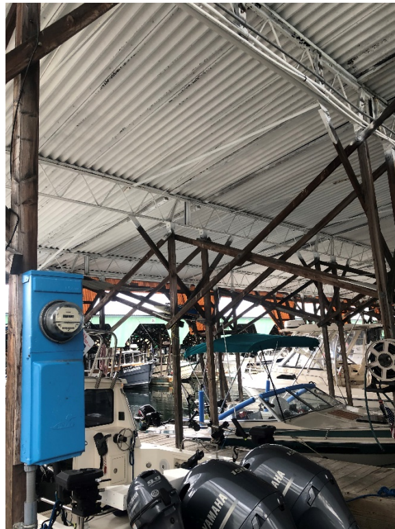
Photo 18. Electrical Service and Painted Truss
