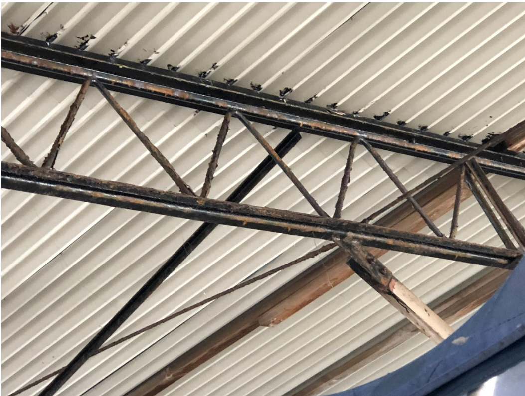
Photo 8. Roof Truss Corrosion
