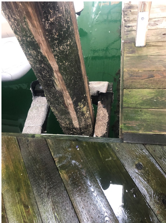
Photo 12. Timber Pile with Abrasion
