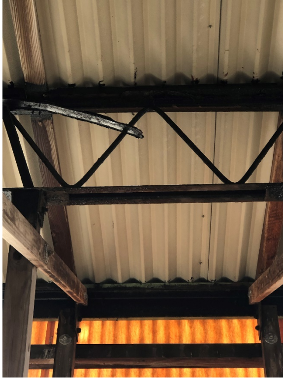
Photo 9. Roof Truss Damage
