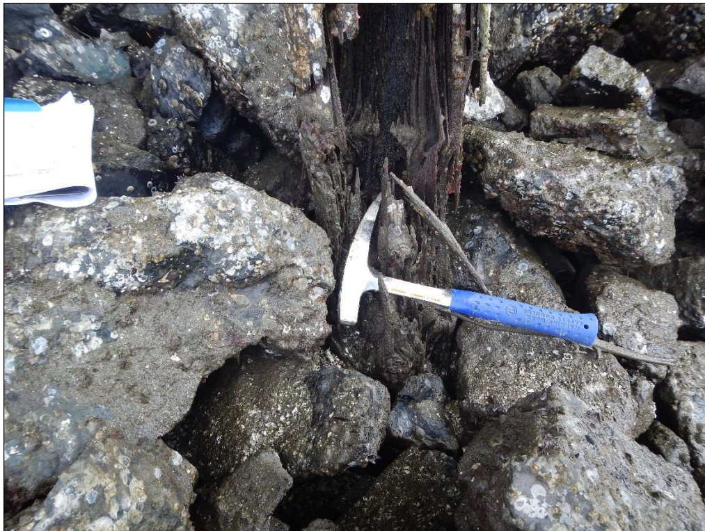
8. Rot through entire pile, 4' high starting at ground line, Bent B Pile C.
