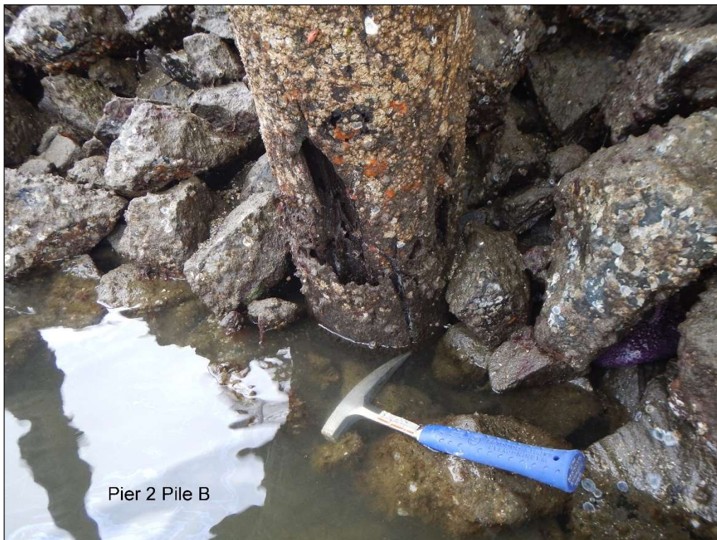
6. Void 12" high x 8" wide x 6" deep starting from the ground line, Pier 2 Pile B (Batter Pile).
