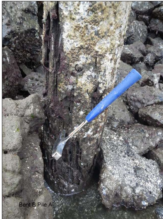
7. Void 24" high x width of pile x 4" deep starting at ground line, Bent B Pile A.
