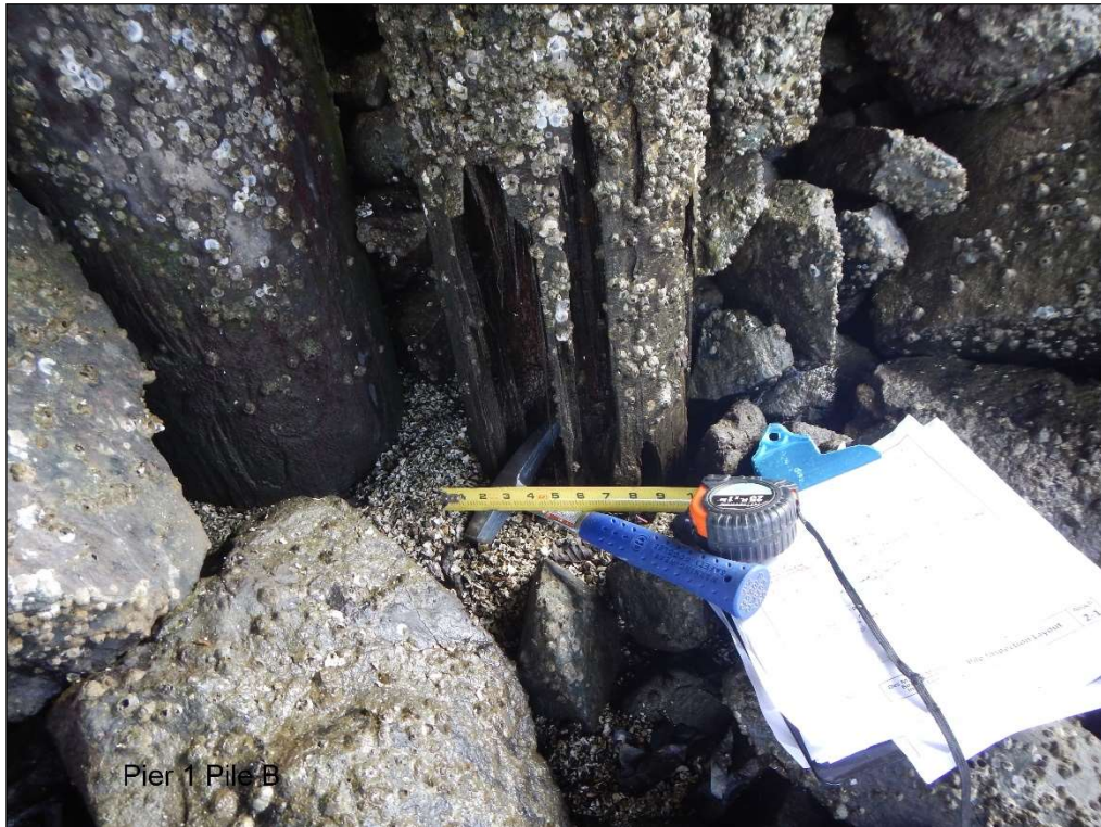
5. Void 16" high x width of pile x 6" deep starting from the ground line, Pier 1 Pile B.
