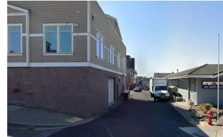
Utility undergrounding completed in Des Moines Theater alley at S 223rd St.
