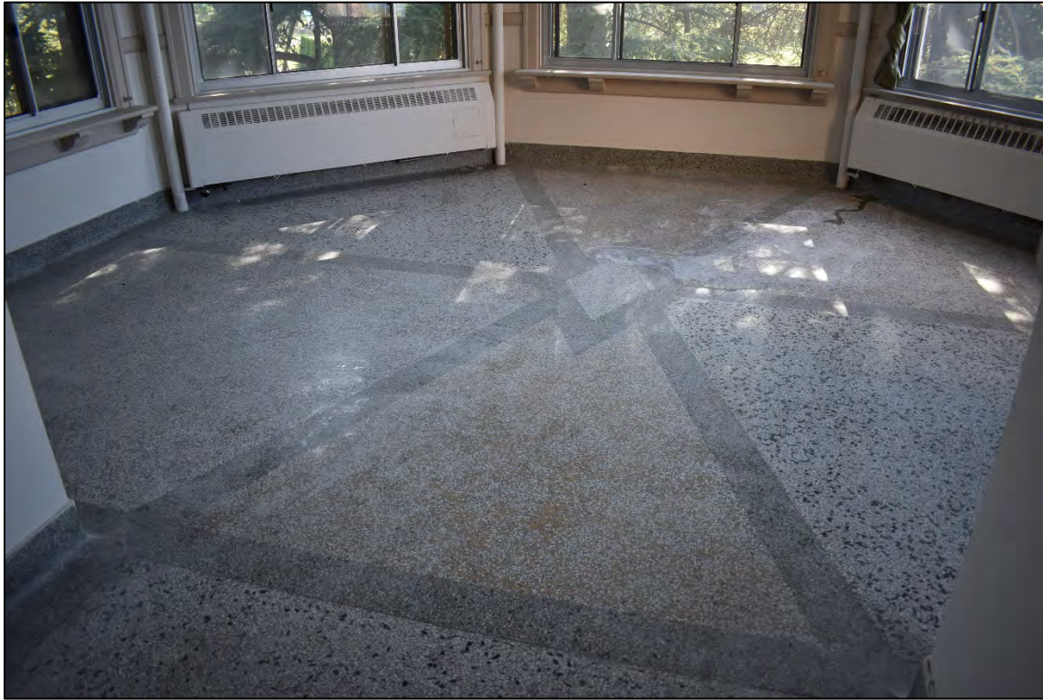
Fig. 82 – Main Building, interior, upper floor, typical solarium at end of residential corridor, showing terrazzo floor.
