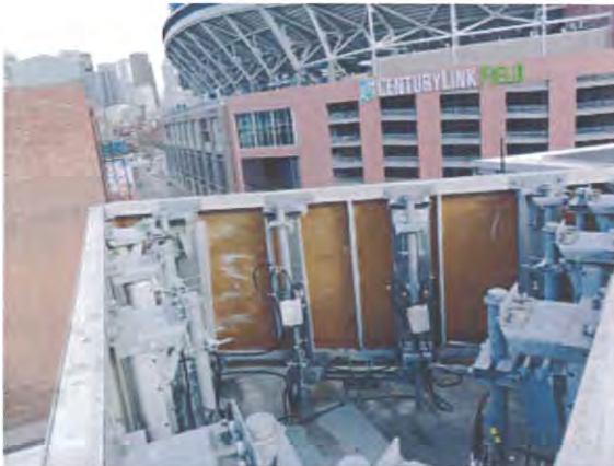
Screening of roof-mounted antennas, and equipment should be integrated into the design of the building
