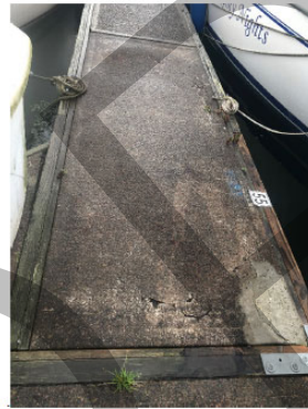
Photo 15. Outer Concrete Float Showing Deterioration
