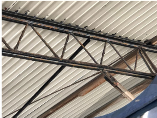
Photo 8. Roof Truss Corrosion
