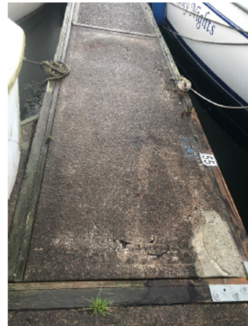
Photo 15. Outer Concrete Float Showing Deterioration
