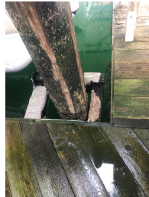
Photo 12. Timber Pile with Abrasion
