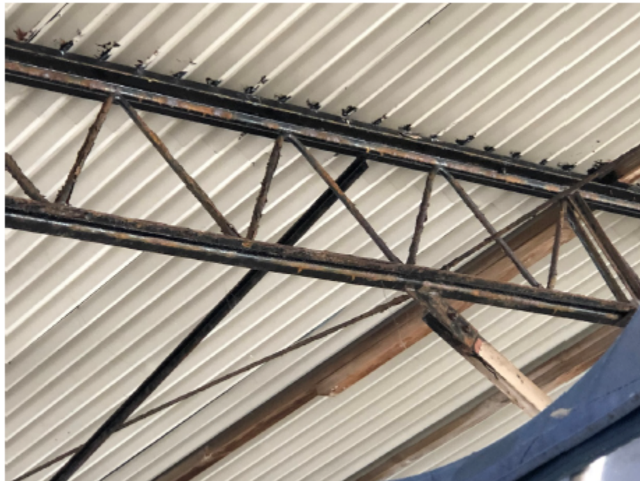
Photo 8. Roof Truss Corrosion
