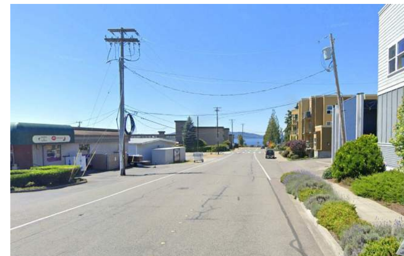
Overhead utility lines just east of S 223rd St and 7th Ave S intersection
